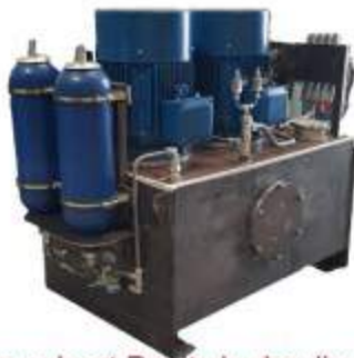
Rescue boat Davits hydraulic units
